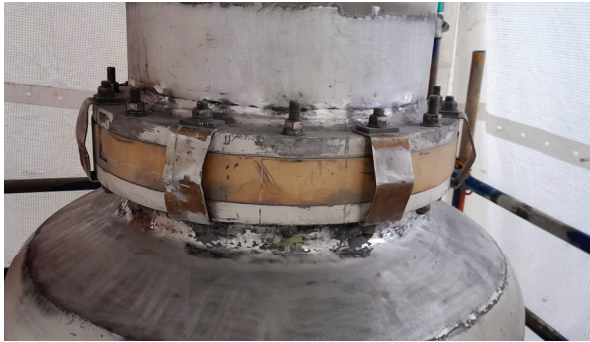
Flange leaking SF 6 gas
