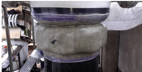
Belzona 7311 applied to breather membrane with Belzona 9341 incorporated. 5x layers of Belzona 9371 utilising Belzona 1981 resin
